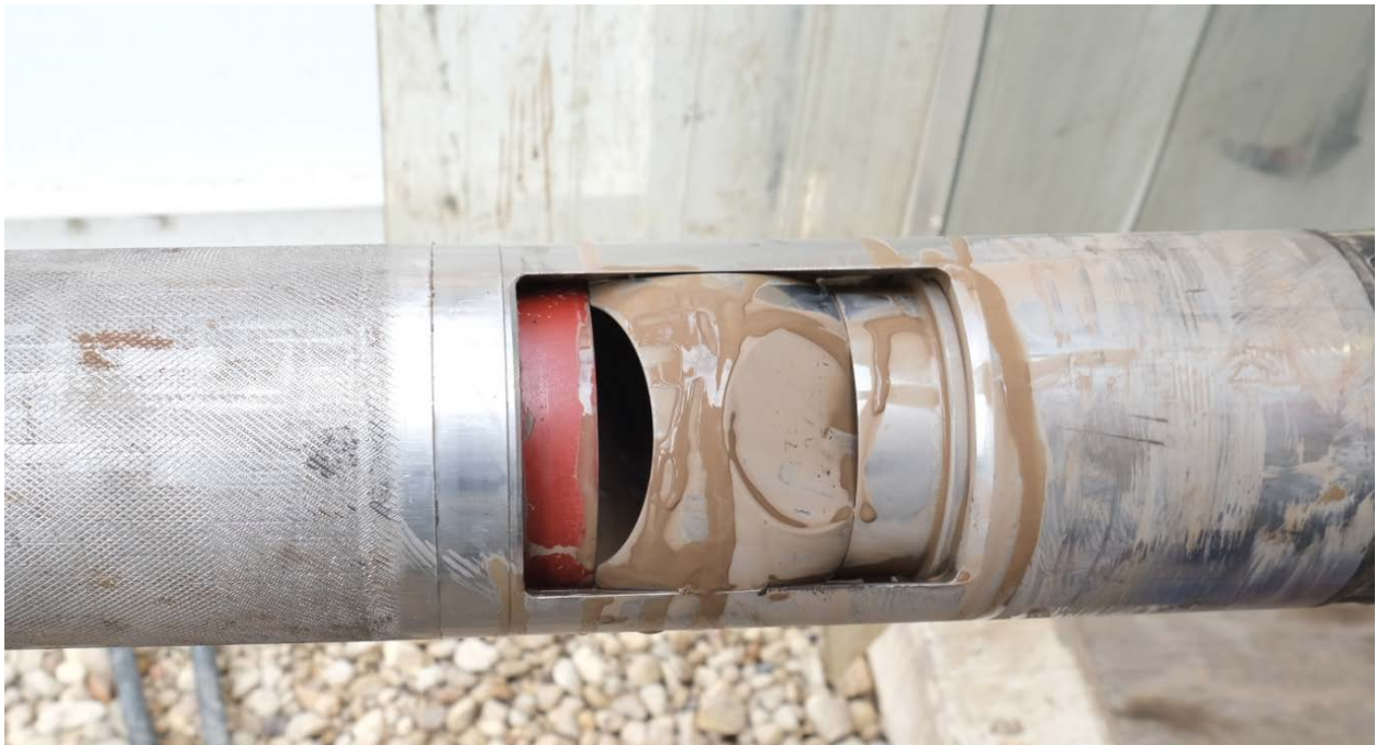
Figure 1: Image of a partially closed ball valve.
