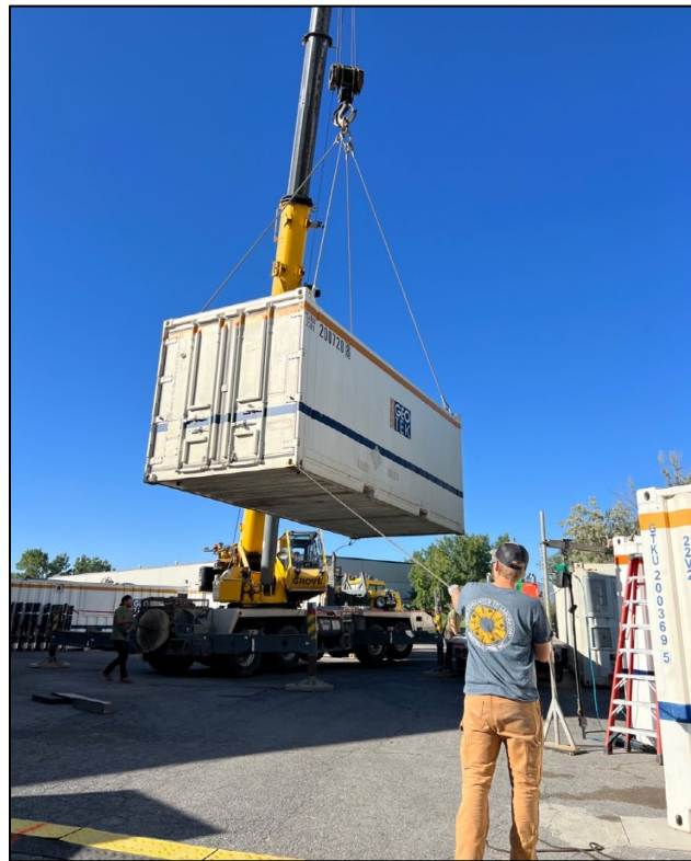
The final container unit with all the cores arrived at Geotek Coring in SLC
